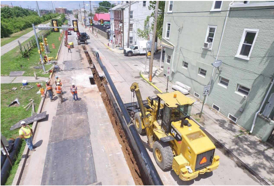
Exelon's gas utilities are focused on actions to reduce operational GHG emissions, including replacement of older cast iron and bare steel gas distribution pipes to reduce trace amounts of fugitive methane emissions. (Photo taken prior to COVID-19 pandemic.)
