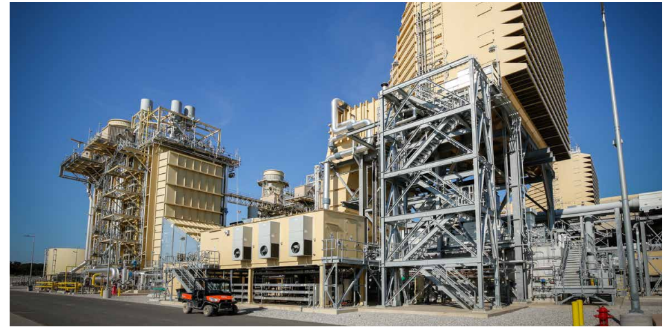
Exelon Power's 1,115 MW Wolf Hollow II state-of-the-art combined cycle natural gas power plant, Granbury, Texas, utilizes the latest pollution control and air cooling technologies.
