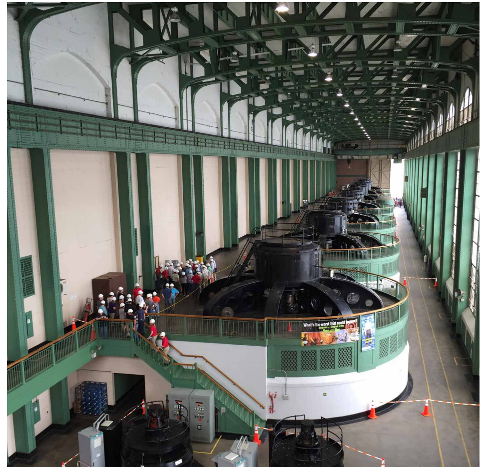
Pre-pandemic community tour at the 572 MW Conowingo Hydroelectric Dam, Darlington, Maryland.
